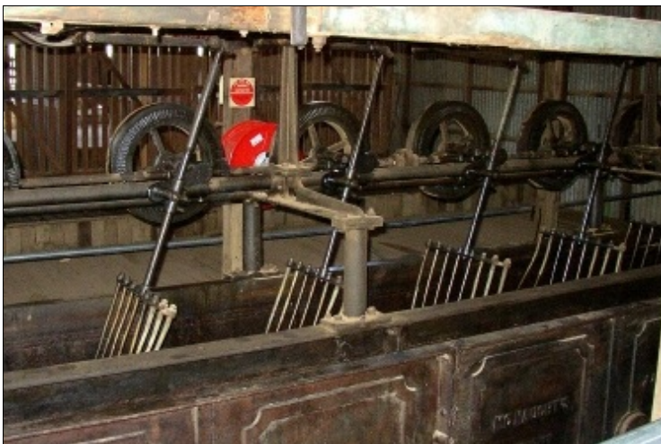
Detail of the original 1908 McNaught scour line.
