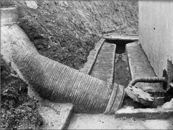
The bottom wood stave pipe fixed to the Port Kembla made cast-iron manifold entering the Power House. Photo courtesy Norman Brown.
