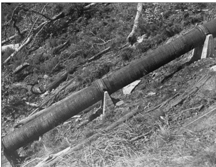
Part of the finished pipeline, showing the pipe collars bolted down to the 31° concrete anchor blocks.
