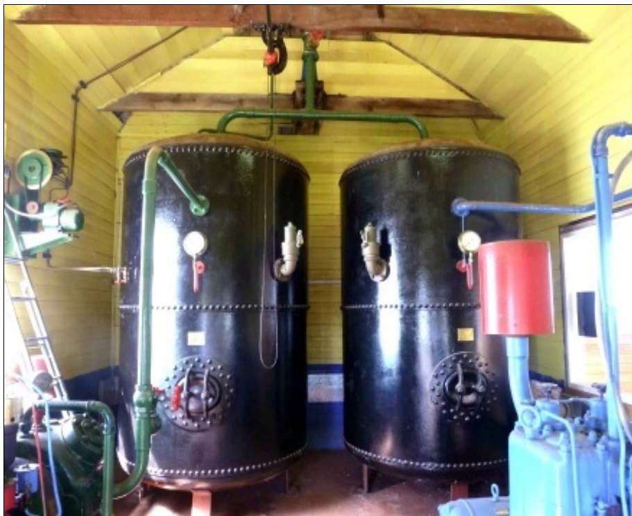
The two air receivers in the foghorn shed, with the timing device on the wall at upper left.
