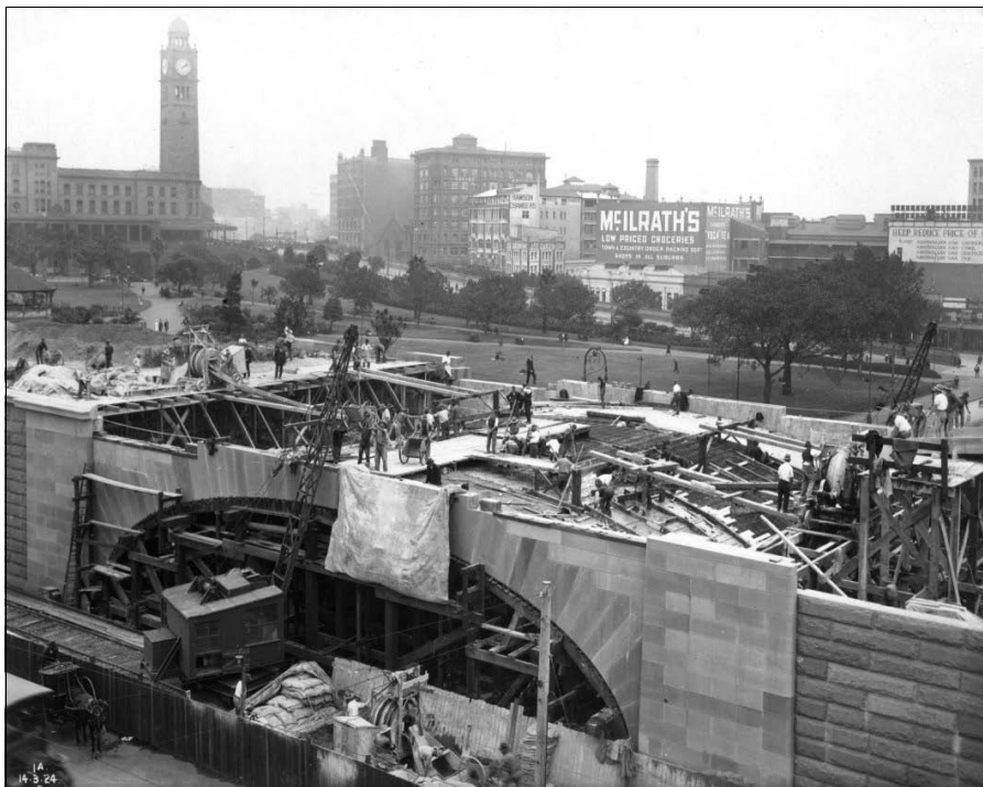
Concreting the arch over Hay St on 4 th March 1924. Electric concrete mixers on platforms over each of the abutments send concrete mix down chutes, while a crane on rails serves a third mixer at street level on Elizabeth Street. Image: ARHS Railway Resource Centre collection.
