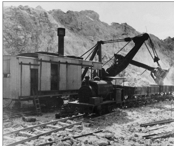
Image left: Bucyrus 65 ton rail mounted excavator serial No 506 loading waste into 3ft 6in gauge Aurora side-tipping trucks hauled by a 10 ton Hunslett loco. Seale Collection.
