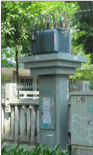
Above: A newer style "pedestal" substation in Hanoi.
