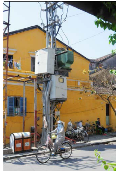
Above: Traditional pole type distribution substation in Saigon.
