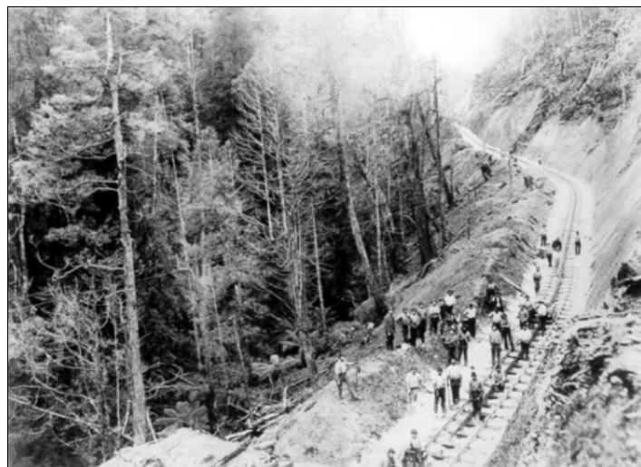
Men working on the Abt Railway in the 1890s Source not attributed - Possibly Tasmanian Archives Office
