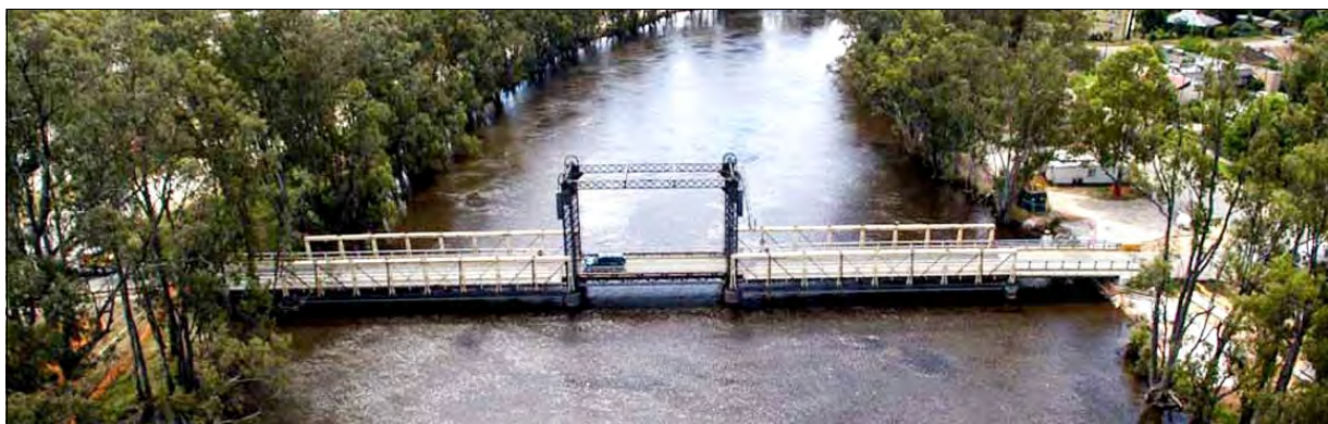
The Barham Bridge after restoration was completed. Photo source: Transport for NSW.
